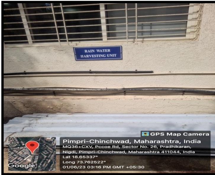
Rain water harvesting system
